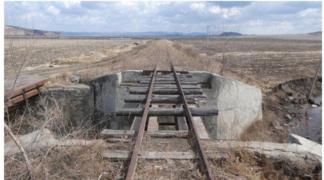
Another bridge needing repair
