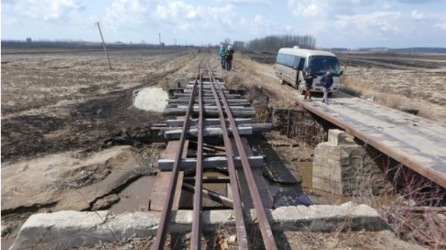
Bridge in need of repair
